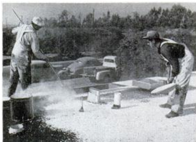
Roof panels in the slab-door house are topped by roofing paper, tar, insulating aluminum foil and final coat of crushed gravel
